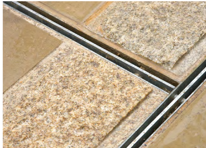
Stainless steel slot drains
